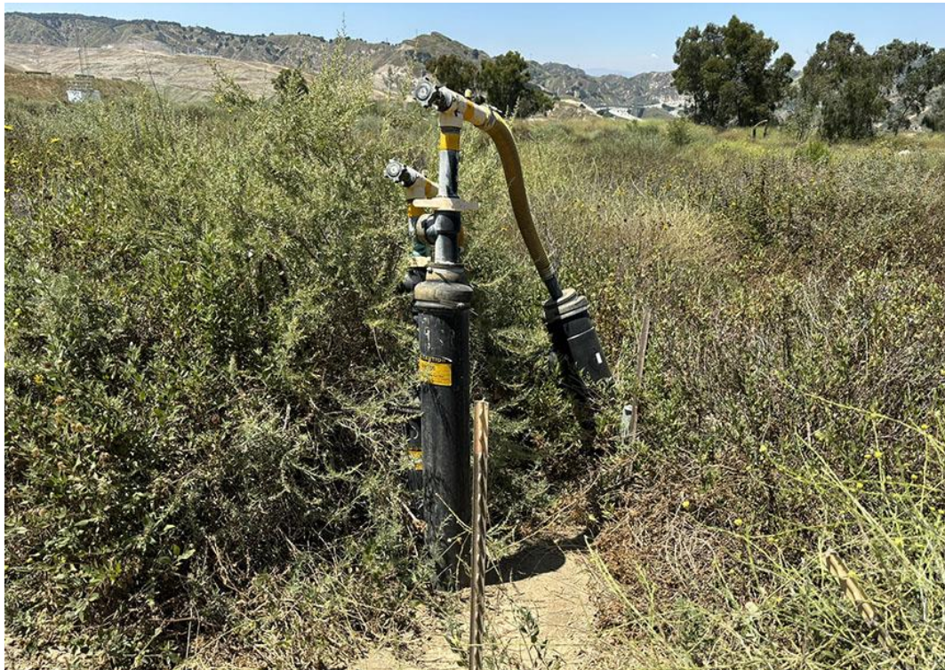
Gas Well with Saltbush growing into clearance zone
