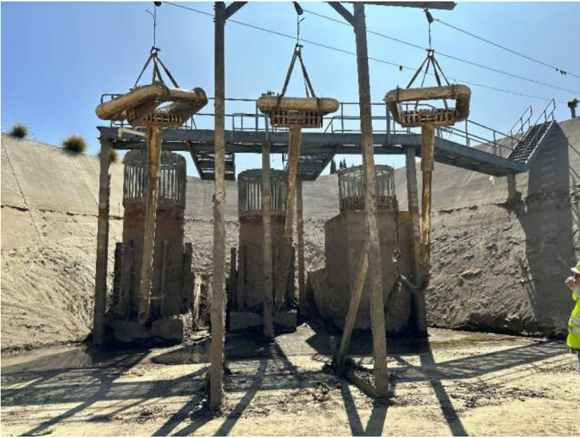
Skimmers, connections good and winches work
